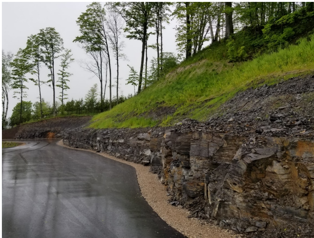
Figure 18 Photo of shale wall taken on June 10, 2019 after scaling and removing the loose debris.
