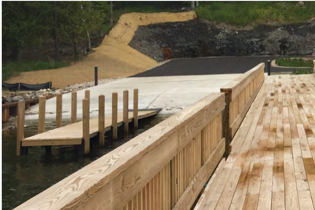
Photo # - Gap in Pier Guard Rail
